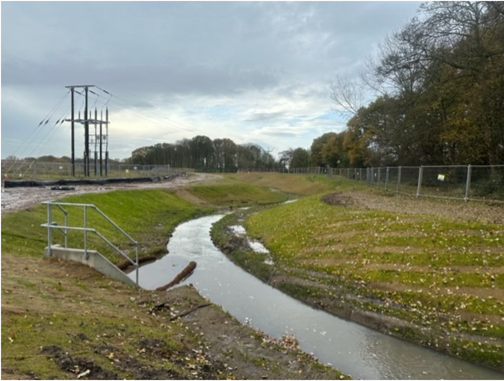
View towards the plot for Unit 4 with diverted brook to the right.
